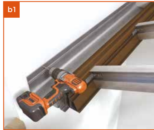
b1 Please ensure you use suitable fixings determined by the wall construction.
