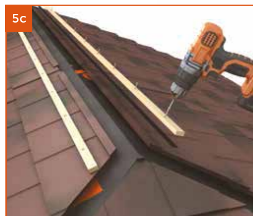
Fit timber battens and screw into place (battens must be kept dry).
