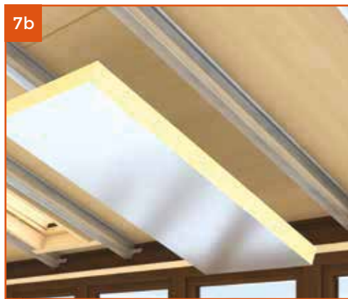
Fix 70mm insulation board between the rafters. The 70mm insulation board should sit flush with the underside of the rafter.
