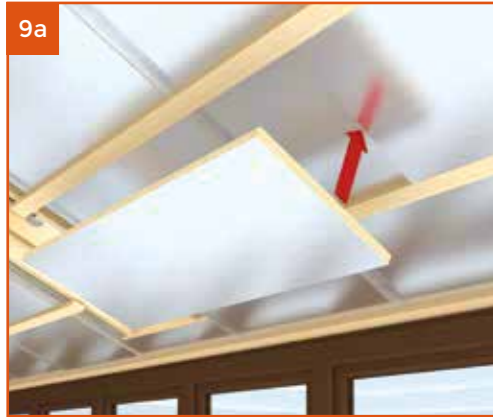
Install 25mm insulation between battens and apply expanding foam to the spider assembly.
