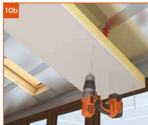
Cut and mitre 82mm insulated plasterboard, fix into position at no more than 50mm in from the corner and at no more than 200mm centres with fixings supplied.
