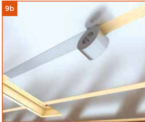
Insulation tape should be run over every batten and the window line so no timber will be visible from the inside.
