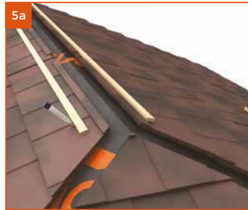
Using the crown ridge and end cap positions as your starter – dry fit battens and ridge profiles to mark out locations.
